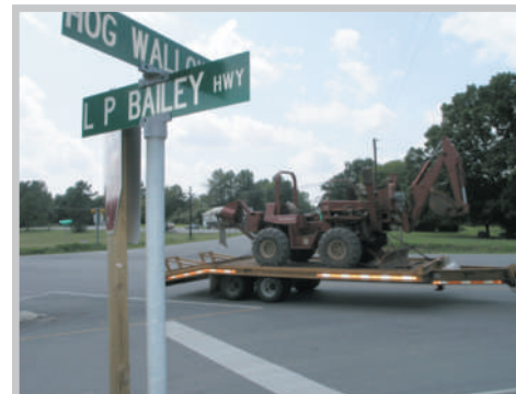
L.P. Bailey highway has been widened to better accommodate two converging routes.
